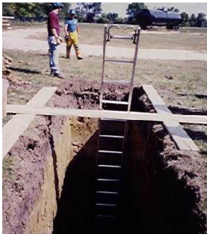
Above: A trench can be a wall collapse, flooding or confined space hazard.
